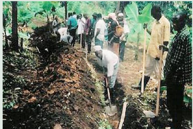
Farmers being trained in the excavation of fanya juu. Soil- and water-conservation measures have led to increases of up to 100 per cent of coffee harvests on the slopes of Kilimanjaro.
